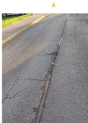
Entrance to Summerfield Road Cracking in road surface
